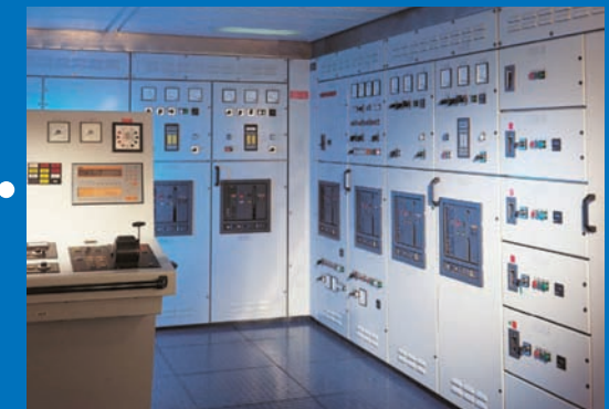
MCC installed in an Off-Shore application with corner section Starters, Distribution Breakers, and Metering
